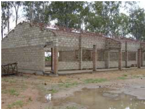
Tiko's first permanent classroom block is taking shape - thanks to a generous private donation from Naperville (USA)
